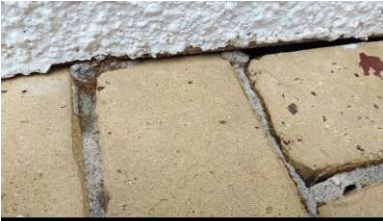
Junction needs sealing.
