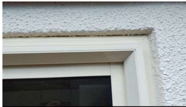
Head flashing not sealed.
